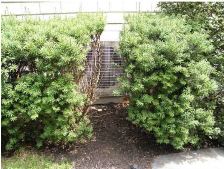
Photo 8-7 Vegetation is obstructing proper ventilation for air conditioning condenser and should be cleared.
