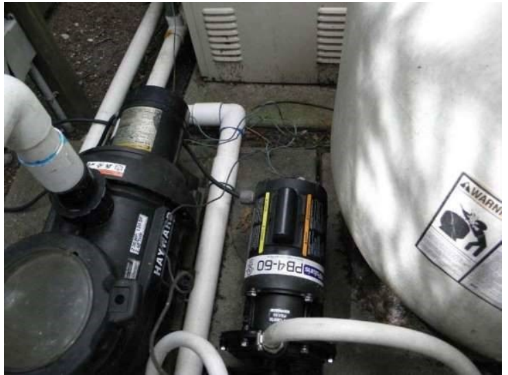
Photo 23-10 Ground wires are connected, but no visible grounding rod appears to be present.
