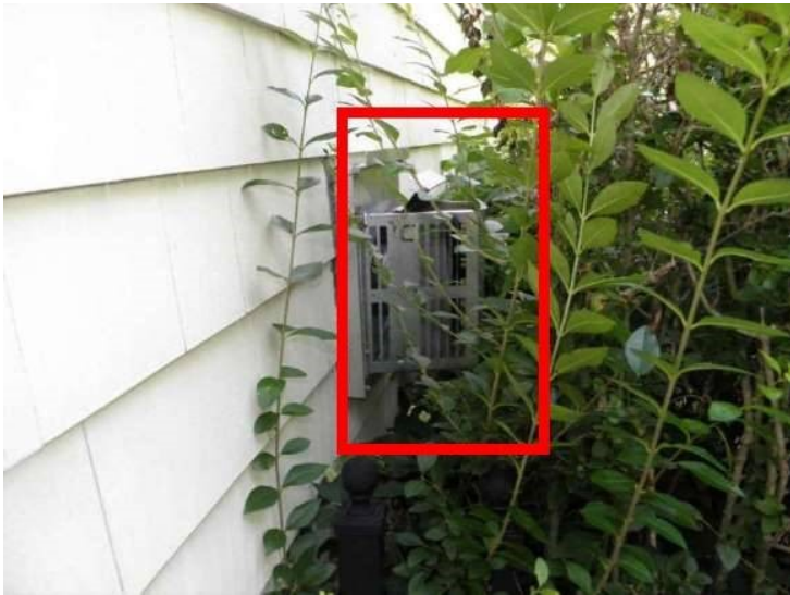
Photo 8-9 Gas fireplace vent should be cleared of surrounding brush.
