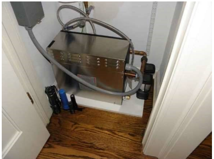
Photo 44-4 Steam system located in hallway closet.
