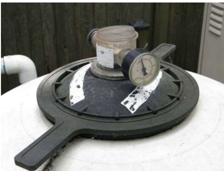
Photo 23-8 Pressure gauge for pool filter
