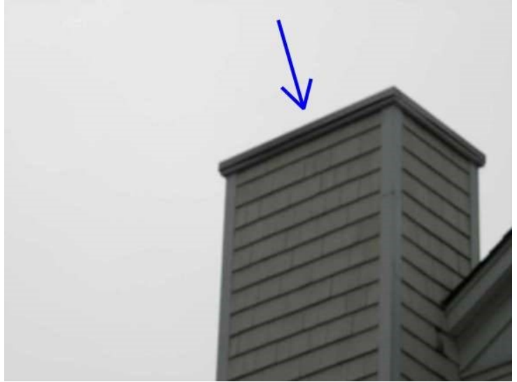
Photo 2-2 No vent on secondary chimney.
