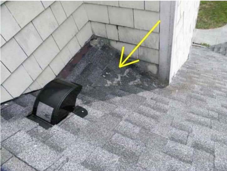
Photo 3-3 Area where possible leaks may occur.
